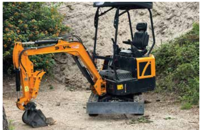
The new digger being put to good use in the construction of the new tee on 8.
